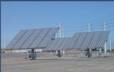
75kW - NV Energy Clark Station Las Vegas, NV
