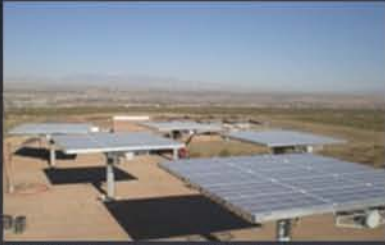
240kW - Southern NV Water Authority Henderson, NV
