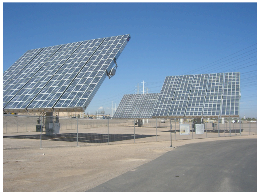
75 kW Amonix Installation at NV Energy
