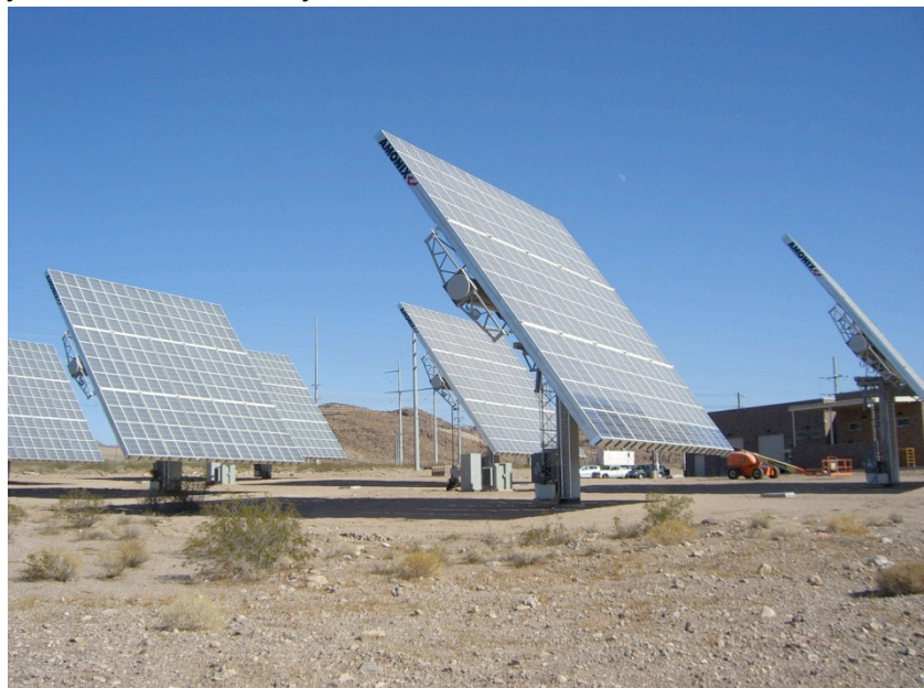
240 kW Amonix CPV Installation at SNWA
