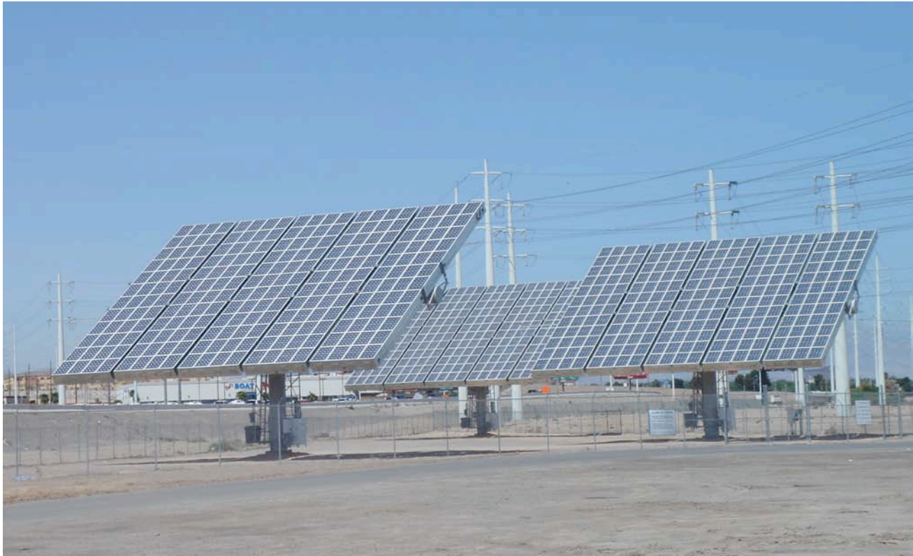
Figure 2. A 75 kW installation for Nevada Power in Las Vegas, Nevada. The systems were installed May 2006.
