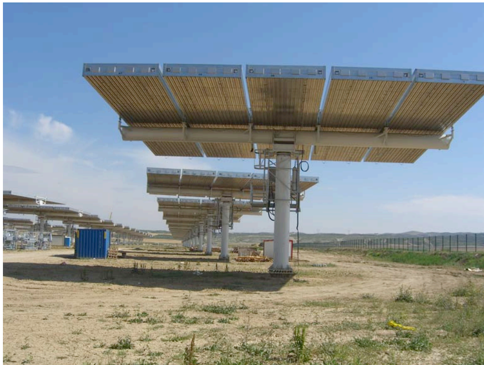
Fig. 4: Guascor Foton's multi-MegaWatt Installation in Spain.
