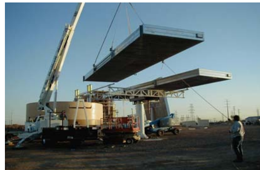
Figure 6. Installation of a MegaModule™. the ground. A 48-inch diameter hole is drilled approximately 15 feet into the ground, depending upon the soil conditions. The pedestal is positioned
