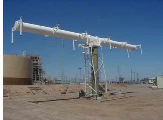
Figure 4. A five MegaModule™ tracking structure.
